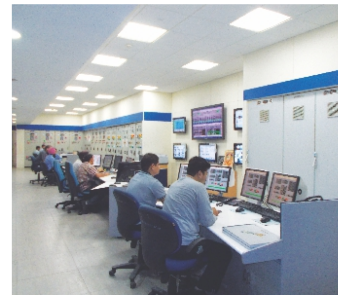
Control Room, Energy Center at DLF Cybercity, Gurgaon
